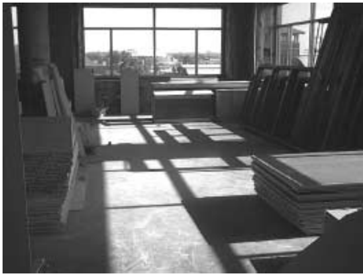
This area of the fourth floor expansion project will be the processing area.
